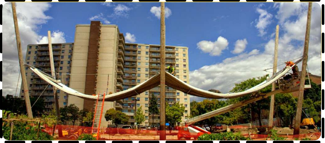
The "Sky-o-swale®" -a green building innovation being patented by the Youth of KGO as part of the Community.Design.Initiative. Image source: East Scarborough Storefront Website
